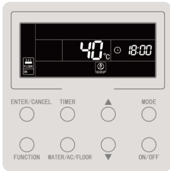
Floor heating on with timer unset
